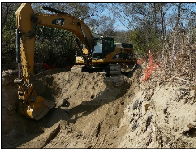
Excavation equipment access areas and haul routes are carefully planned to optimize efficiency and minimize impacts to habitat.
