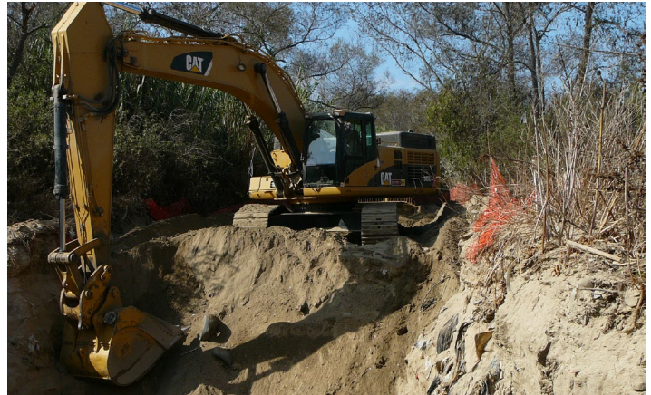
Periodic excavation of channel conveyances to reduce flood risk requires cost-efficient sediment reuse and disposal options.
